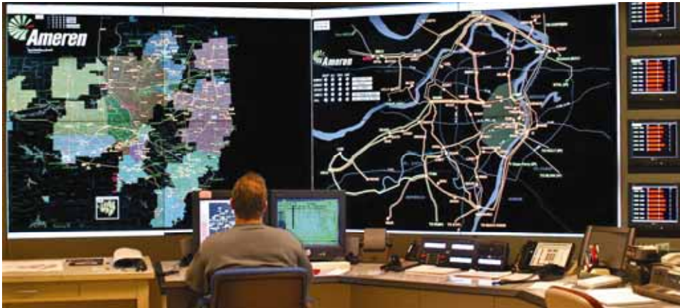
Control room display from Clarity Systems
