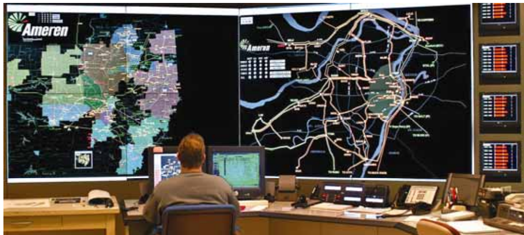
Clarity multi-panel display at utility control center.
